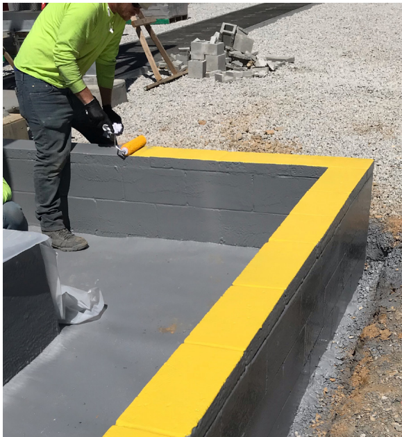
Full secondary containment with GC-2100 liner material and SC-3900 coating spray applied to a transformer pad.
